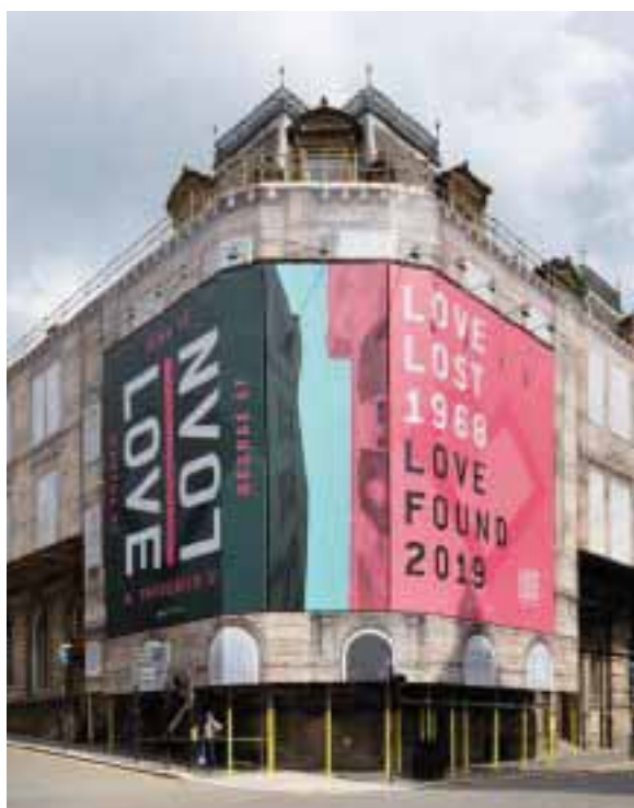
Above: Work has begun on the Chris Stewart Group-developed plan for a 245-bed AC by Marriott hotel, part of a £100m mixed-use development which will transform the north east corner of Glasgow’s George Square into the city’s newest neighbourhood, Love Loan
